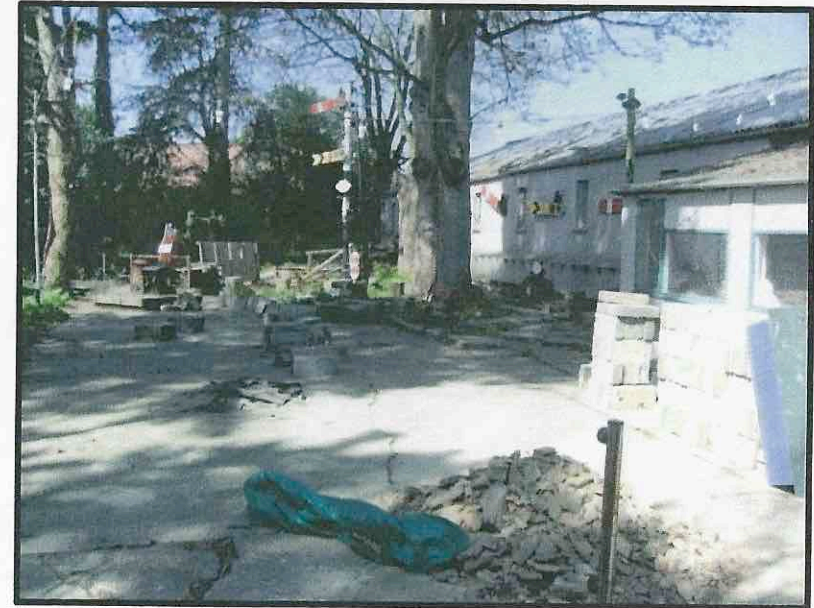
The outside area is being cleared, ready to start building the new portable layout.
