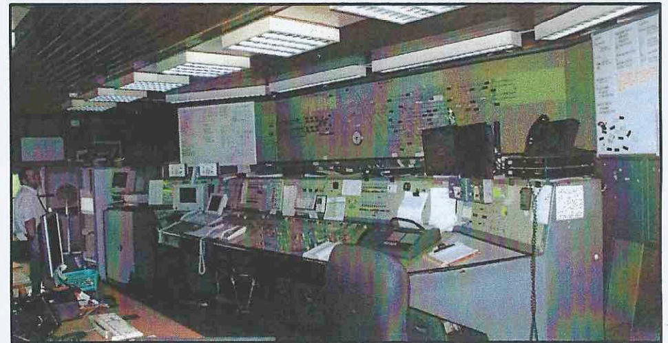
General view of the control room
